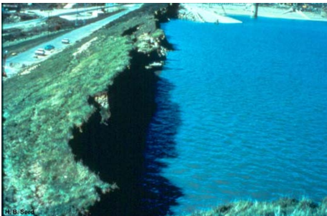
Figure 4 A close-up view of the slide head scarp
